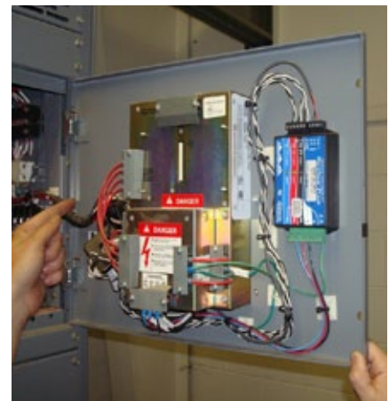
Installed Energy Management System
