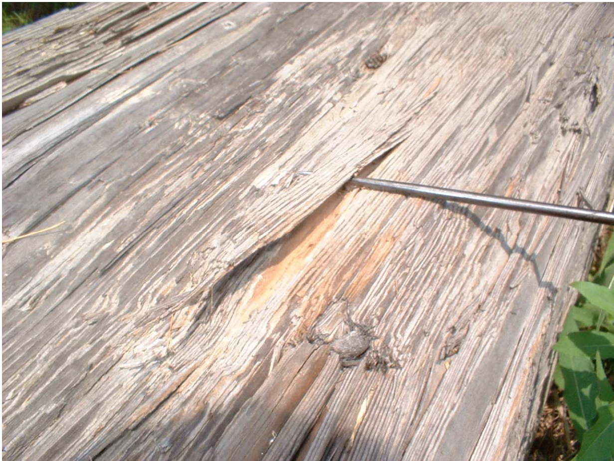
Figure 1a. When subjected to the “pick test” this sample broke in a single, solid piece far from the tool. It was difficult to penetrate deeply, and the wood under the splinter is intact and looks new. The sample is not appreciably degraded by fungal decay and may be considered sound.
