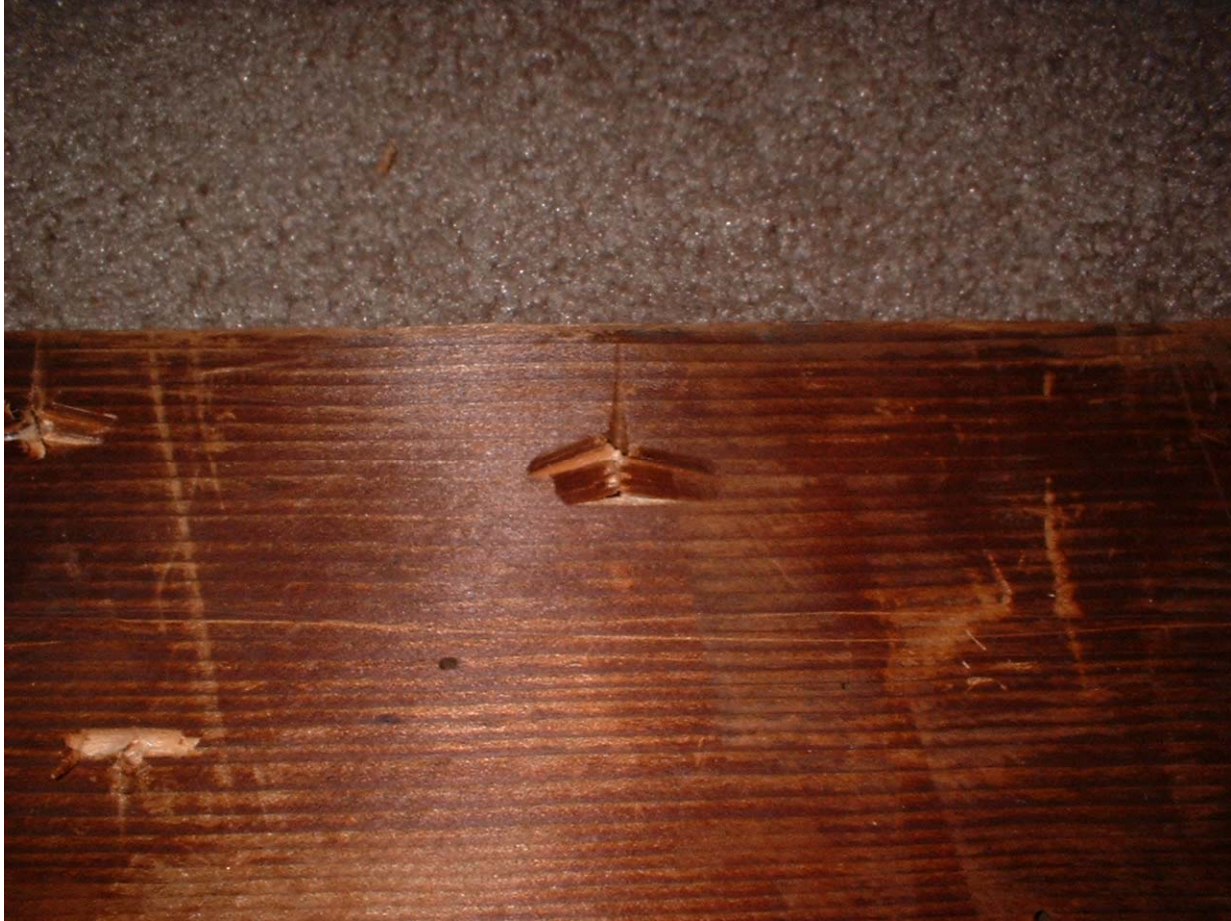
Figure 3. On its surface, this 50-year-old Douglas Fir purlin looked sound. When subjected to the pick test, however, decay is indicated by a brittle cross-grain break directly over the tool. The entire break is less than 1-inch (25 mm) long.
